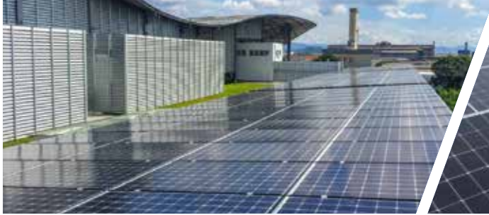
Solar panel at UOM
